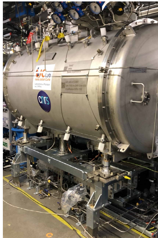
Figure 4: Medium Beta CM (top) and Spoke CM (bottom) of the pilot installation in the ESS tunnel.
