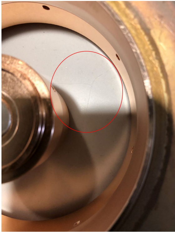
Figure 6: PPU coupler failure during conditioning.
