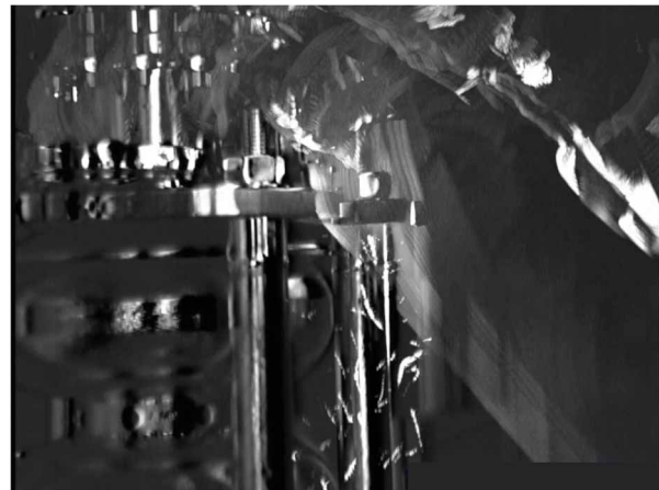
Figure 2: Release of bolts of blind flange using a hex key and hands. Composite picture of a 15 second video.
