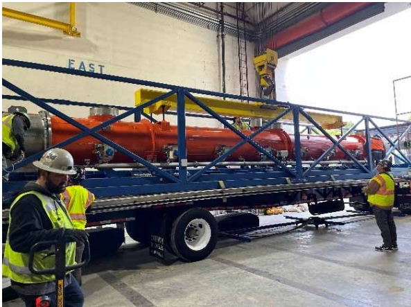
Figure 1: Cryomodule unload in storage area.
