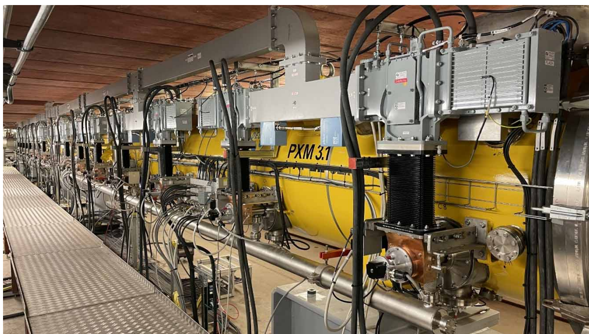
Figure 5: Module PXM3.1 installed in FLASH.
