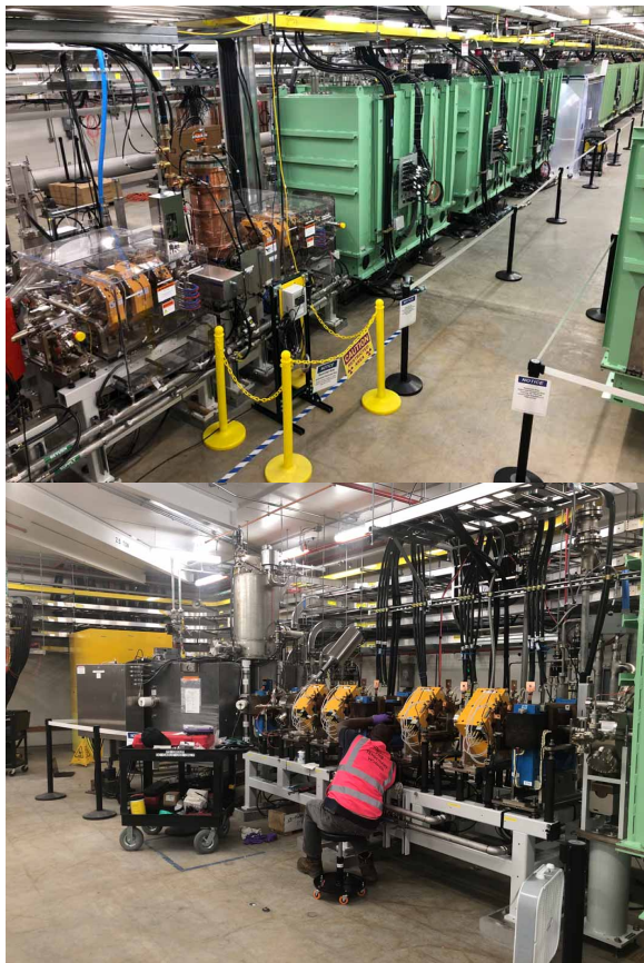
Figure 6: (Top) White tape barriers around the cryomodules in the Linac Tunnel during the installation. Only trained and authorized workers have access inside the white tape barriers – Beamline Limited Access Area. (Bottom) Workers must wear a pink vest when working in the Limited Access Area.
