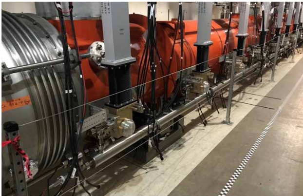
Figure 1: Cryomodule installed in the SLAC tunnel.
