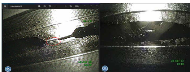
Figure 8: (Left) weld area with non-penetrated weld (break in underbead), (right) weld underbead after repair.
