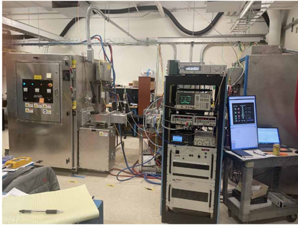
Figure 10: Current magnetrons, unit #1 and #2 installed at LERF, JLab with injection locking and PLC magnetron controls.
