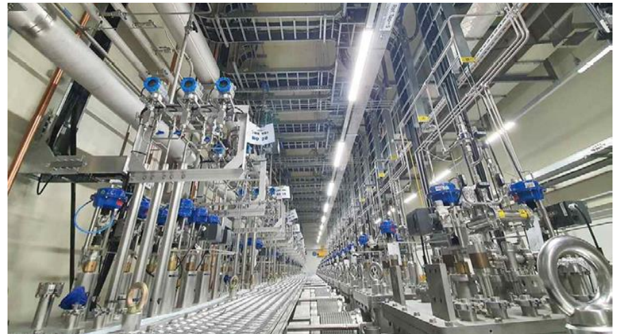
Cryogenic Distribution to Cryomodule
