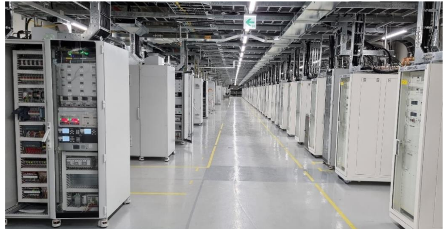
CM/Cryogenic Control Rack and SSPA
