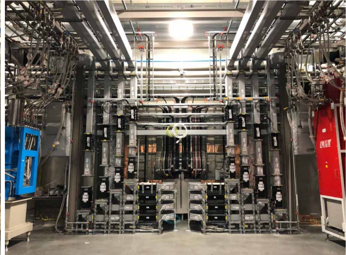
RF waveguides in the klystron gallery
