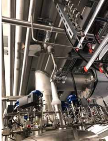
Leaky valve seats
