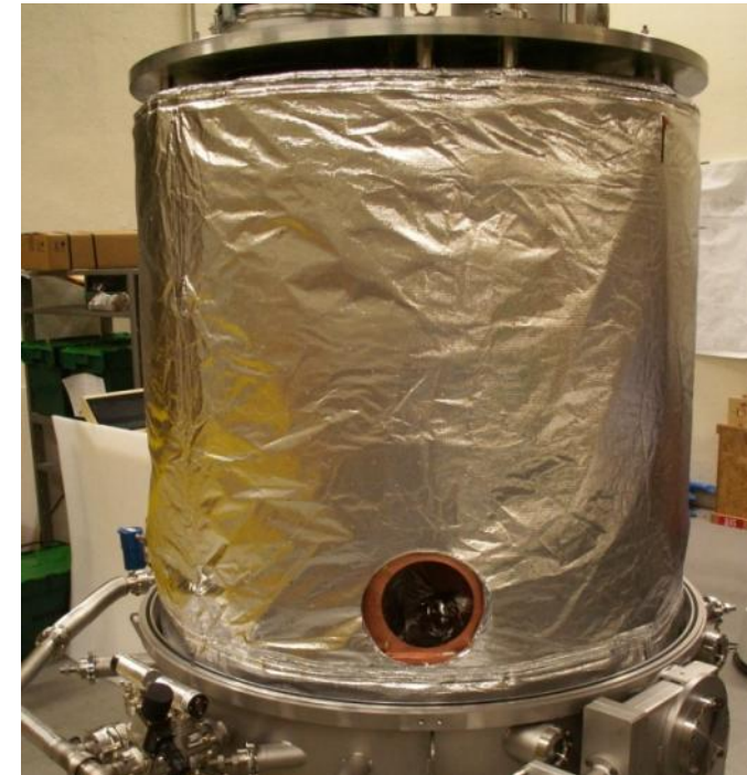
MLI installed on the thermal shield
