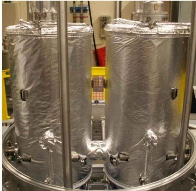
MLI installed on the cold mass: the two QWR and the cryogenic piping
