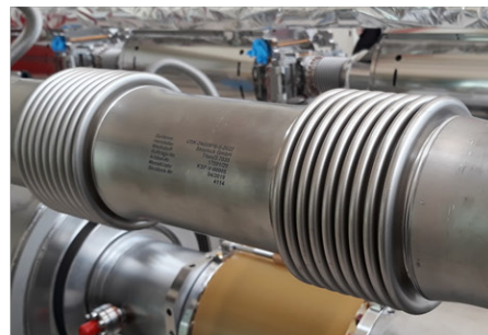
Bellows on the 2-phase pipe
