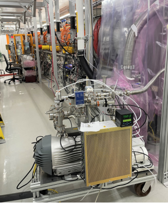
Vacuum cart – connected to Endcap side
