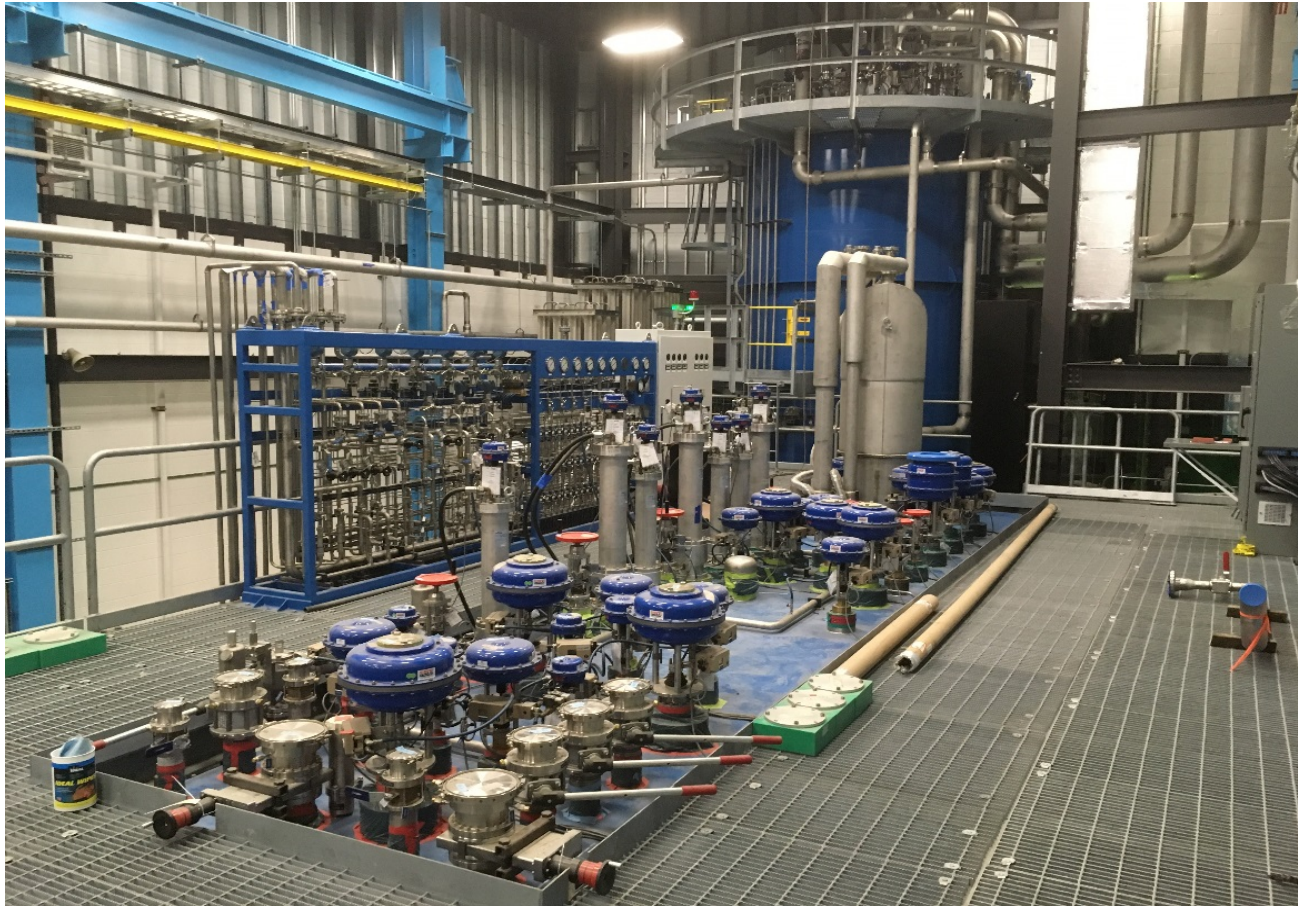
4.5 K helium cold box (upper and lower sections; cold box room)
