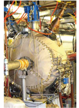
Existing 197MHz NCRF Cavity for Bunch Compression
